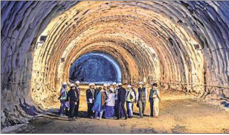
Union Minister for Road Transport and Highways Nitin Gadkari reviewing work on the Zojila and Z D Morh tunnels, in Baltal, Jammu and Kashmir, Tuesday. PTI
