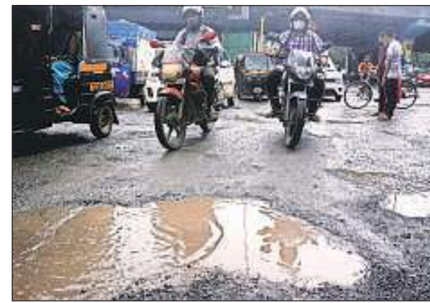
Potholes on Ghodbunder road. Deepak Joshi
